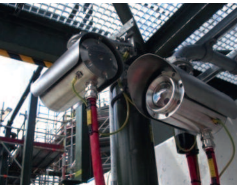
ELDS™ systems installed in field operations
